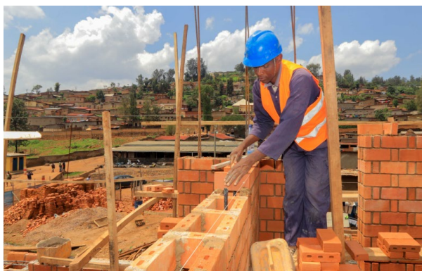
Construction of the Affordable Urban Housing Block for the transformation of the informal neighbourhood of Kigali Kimisagara. (photo: Isaac Rudakubana)
