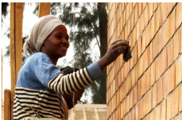
Female construction professional in charge of pointing and finishing of the "smart & green brick walls" of the Swiss Cube building at EXPO 2017. (photo: Daniel Wyss)
